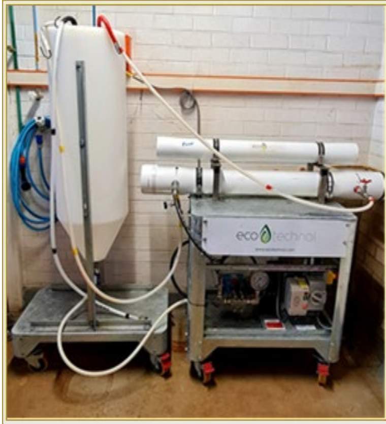
Figure 41. Ultrafiltration / Nanofiltration rig used in this study (Ecotechnol).
