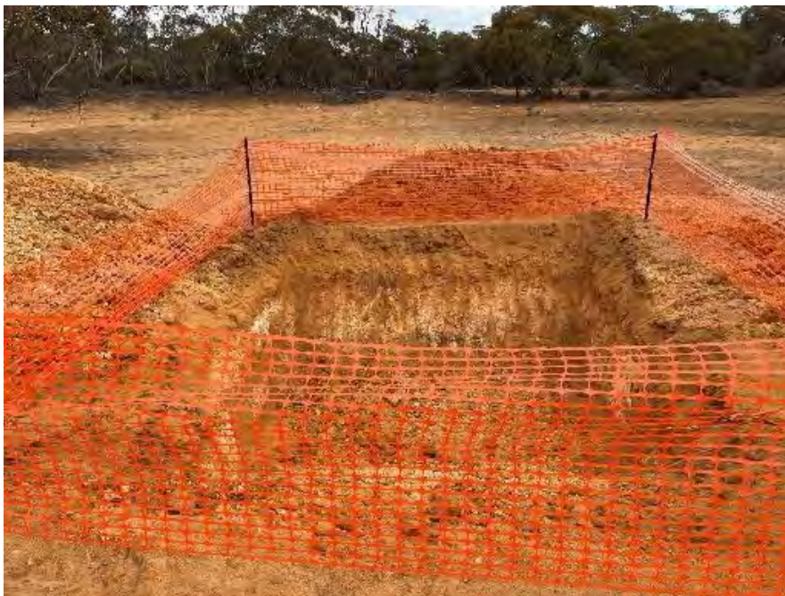
Figure 10. Dry sump constructed in preparation for drilling at the Delamerian NDI campaign.
