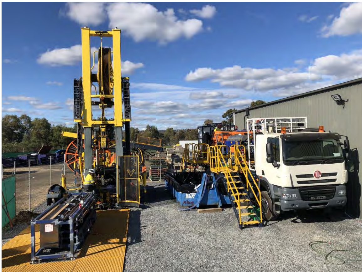
Figure 12. RoXplorer® 500 and HPS set up to drill at the UniSA Mawson Lakes campus.
