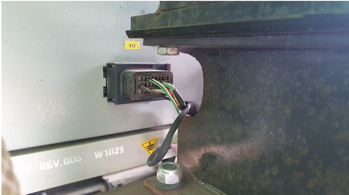
Figure 18: Low Voltage Wiring for Chiller
