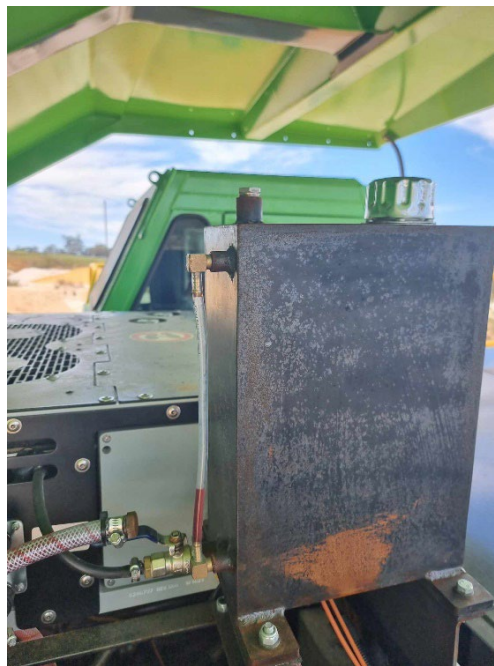
Figure 7: Cooling System Header Tank
